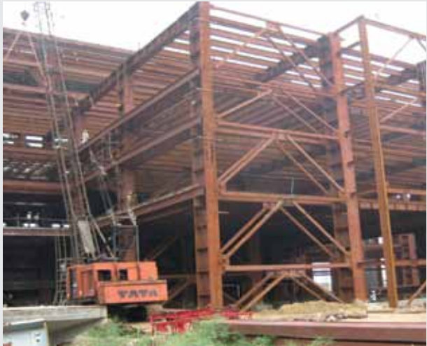
2 X 600 MW North Chennai Power Station, India
