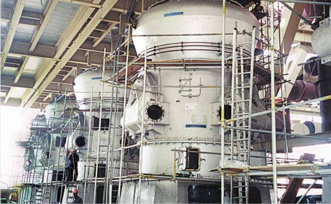
3 X 700 MW Manjung Power Plant, Malaysia - Mill Bay
