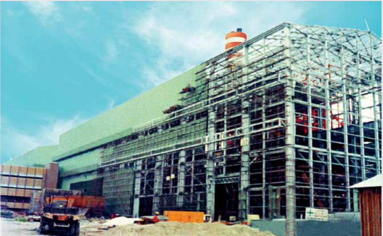
Sultan Salahuddin Abdul Aziz Power Station Phase II & III, Malaysia
