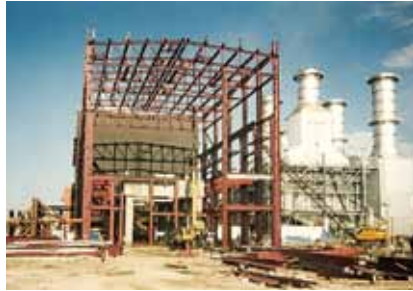
Senoko Power Plant, Singapore
