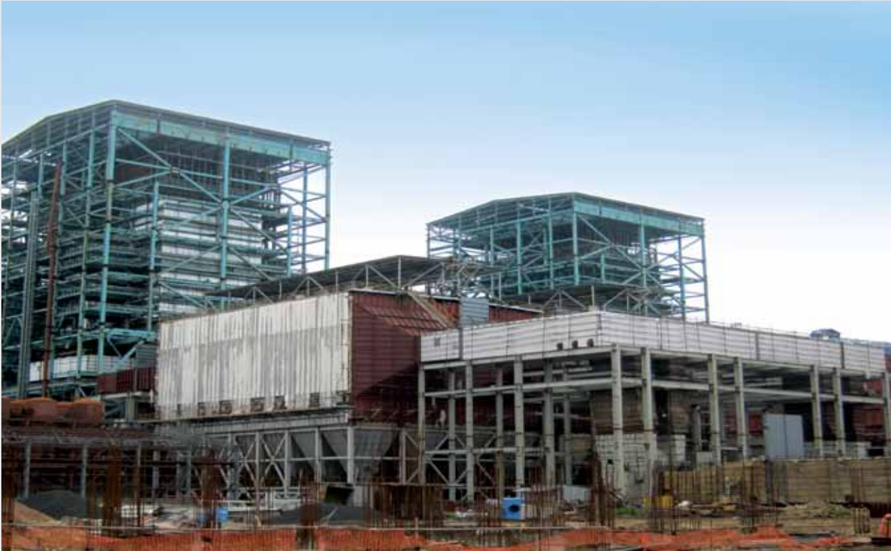
2 X 300 MW EMCO Thermal Power Plant, India
