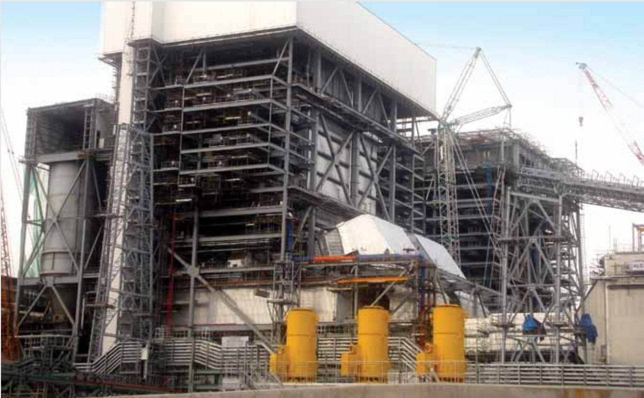
2 X 700 MW Jimah Power Plant, Malaysia
