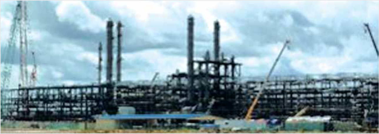
Polycrystalline Silicon Plant, Malaysia
