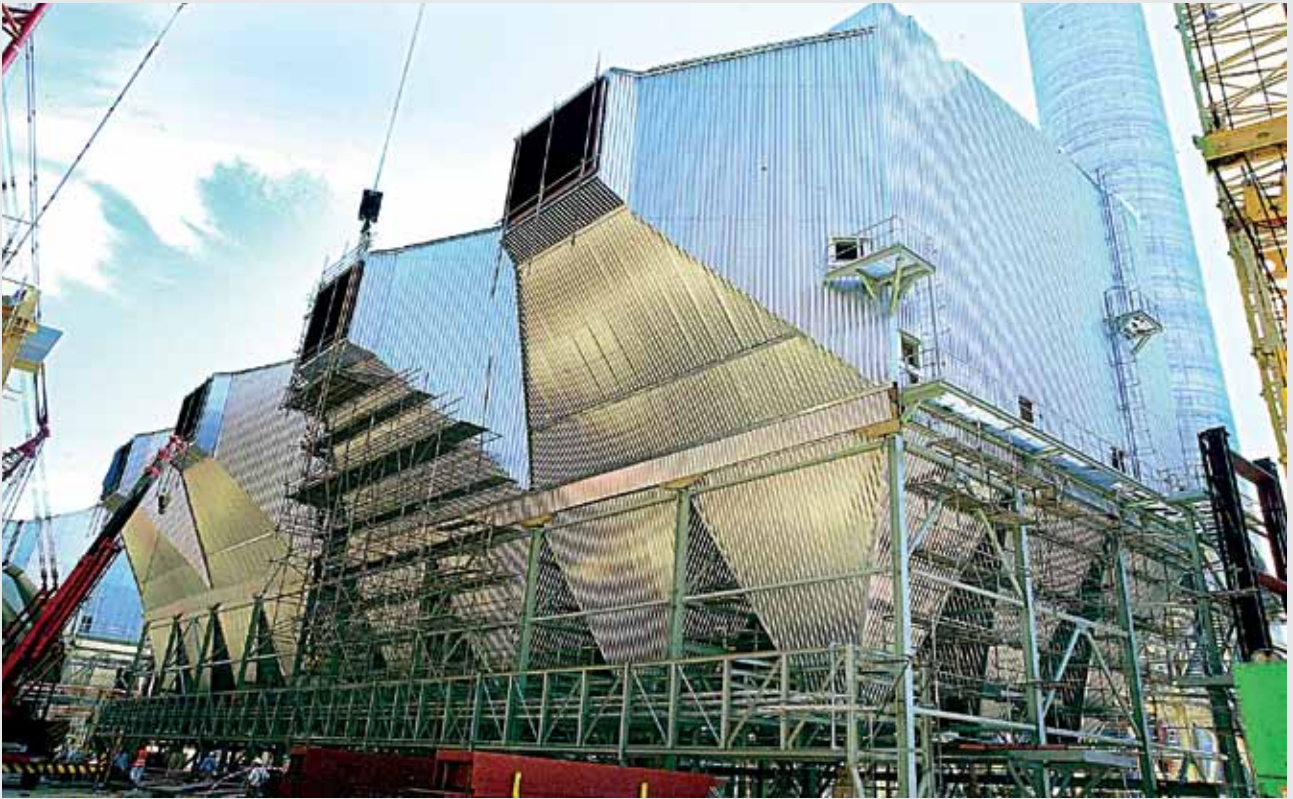
3 X 700 MW Manjung Power Plant, Malaysia - Electrostatic Precipitator
