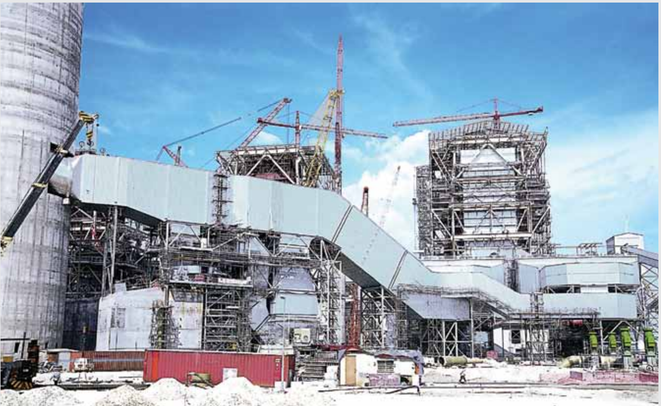
3 X 700 MW Manjung Power Plant, Malaysia - Fuel Gas Desulphurisation
