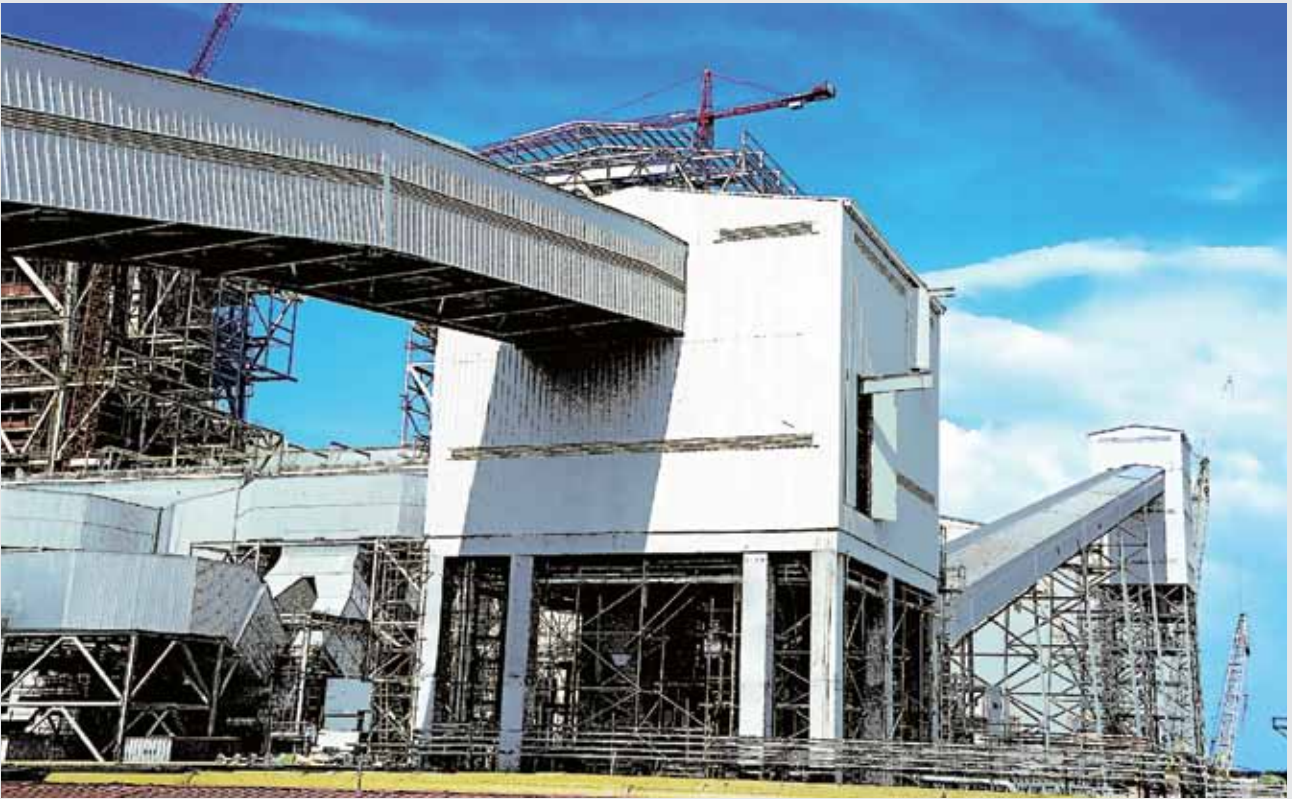
3 X 700 MW Manjung Power Plant, Malaysia - Coal & Ash
