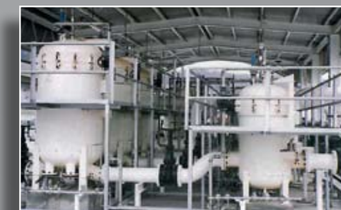
AVIATION FUEL HYDRANT & TERMINALS
