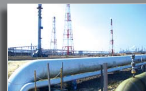
OIL AND GAS PIPELINES & METERING FACILITIES
