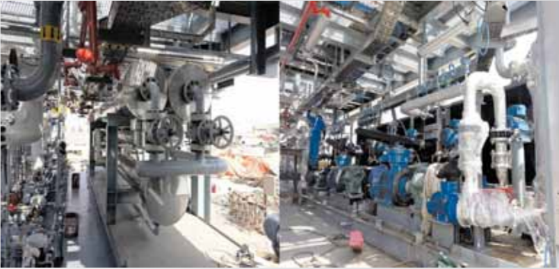
Chiller and MTR
