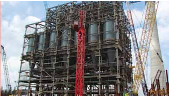
• 1 X 1,000MW Tanjung Bin Power Plant - Unit 4, Malaysia
