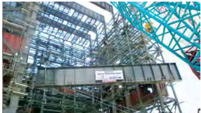
December 6 Lifting of Top Girder weighing almost 200 tonnes at Manjung power plant Manjung, Malaysia
