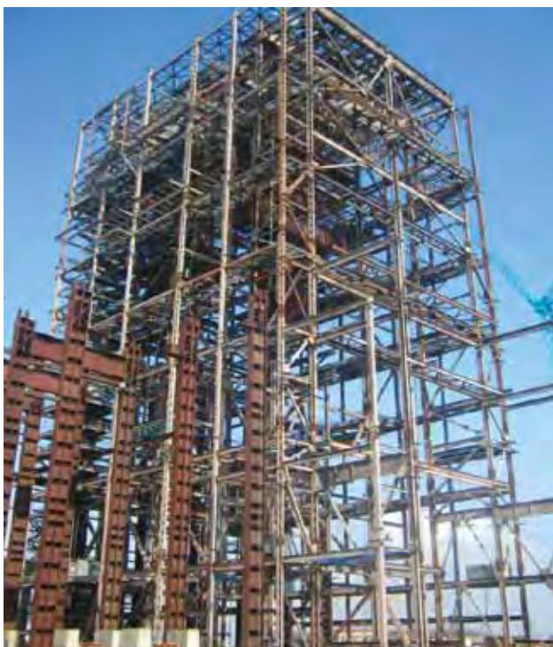
NTPL Tuticorin 2x500 MW Power Plant
