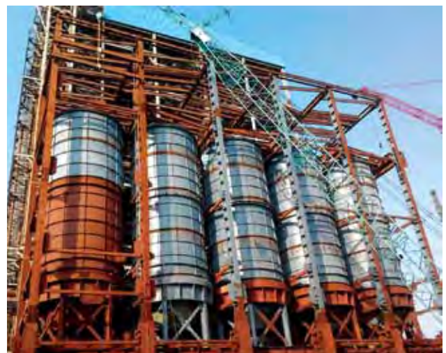
North Chennai 2x600 MW Power Plant
